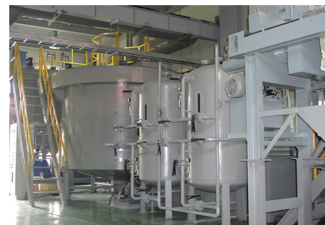
폐수처리장치 _ WASTE WATER DISPOSAL PLANT
